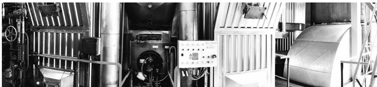
Low-emission gas burner of K1 boiler after denitrification
